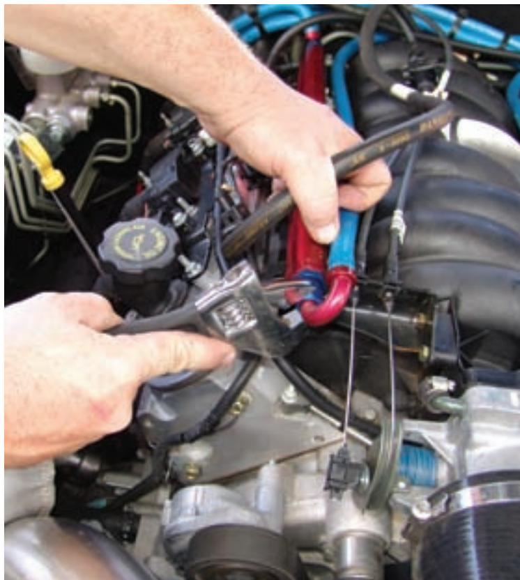
Make sure you tighten all fittings thoroughly after a fuel system install and then check for leaks. Also, make sure you use the right tool for the job, which is questionable in this case!
